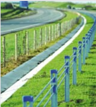
Wire-rope barriers reduce the severity of run-off-road crashes and eliminate head-on crashes from poor overtaking
